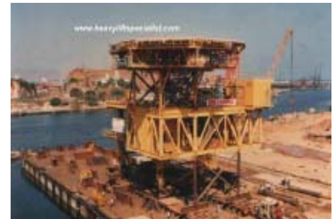
Load-out of 2x700 tons Offshore desk at Hindustan Shipyard in Visakapatnam, India
