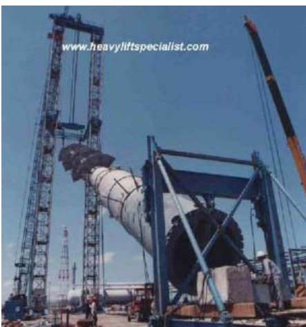
Erection of a 220 Tons column with an unguided lift gantry in Kerteh Malaysia, project was carried out in close co-operation with freight forwarder Kontena Nasional
