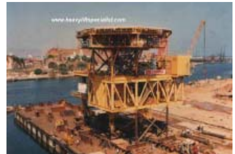
Load-out of 2x700 tons Offshore desk at Hindustan Shipyard in Visakapatnam, India
